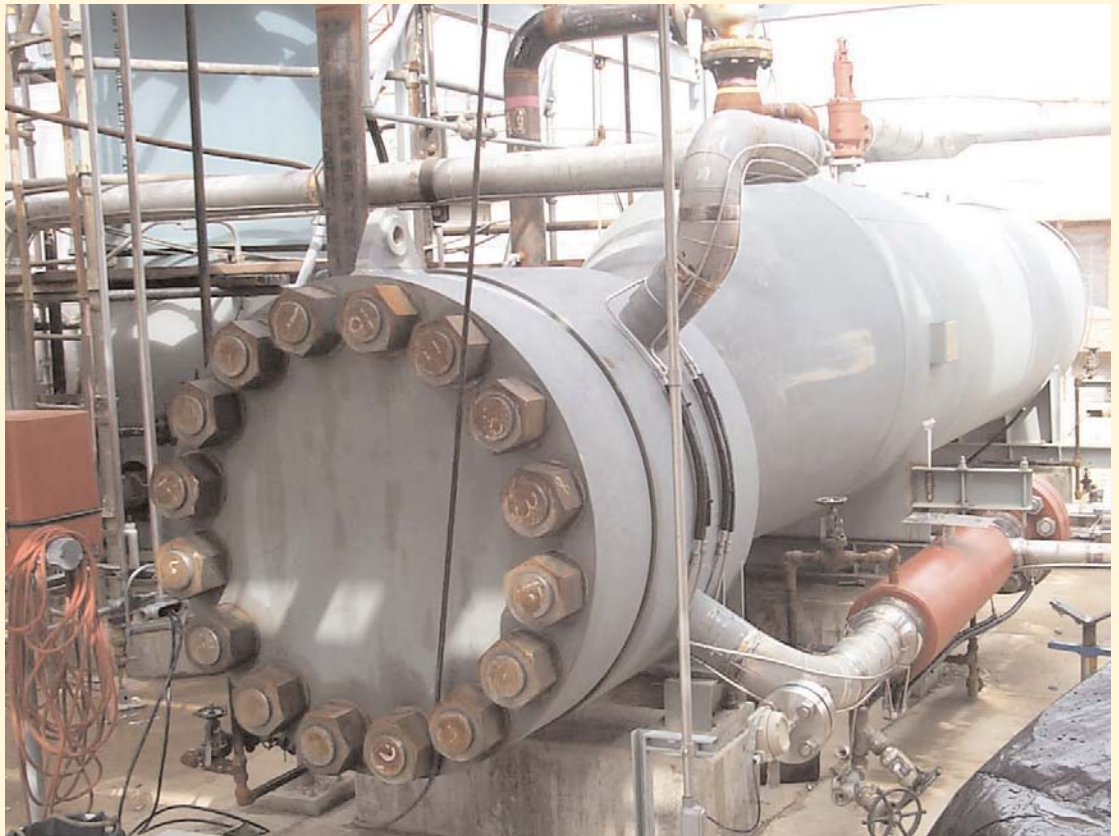
Channel cover plate on primary reactor unit.
